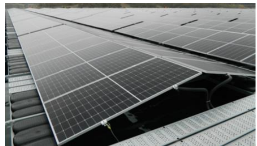
Fig.2: Possible application of a floating PV system © Photo by Welser Profile GmbH
