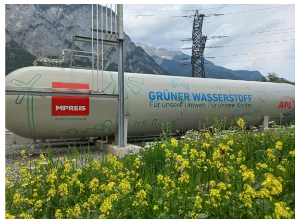
Fig.2 : Production of green hydrogen in Austria using the example of Mpreis. In the electrolyzer, water is broken down into hydrogen (H 2 ) and oxygen (O 2 ) using electrical energy. While the oxygen is released back into the atmosphere, the hydrogen is stored under pressure. This can then be used as a valuable fuel. Only green electricity, primarily PV electricity, is used for electrolysis. The electricity generated from hydrogen supplies energy for trucks and the company's bakery, among other things.
